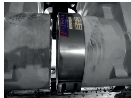
Connection of pipes in an industrial plant.
